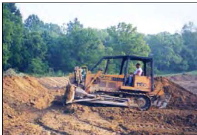
Dozer packs soil in layers to build a dam above the core.
