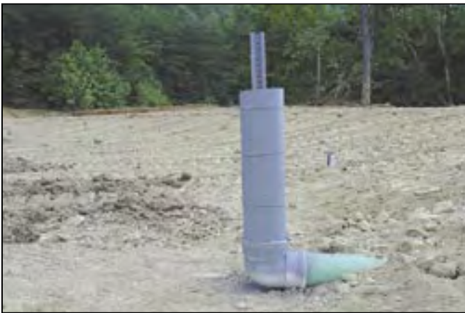
This PVC pipe serves as an overflow pipe when vertical; the stake provides support to the pipe.
