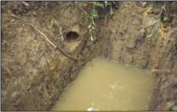
The core will crush buried drainage tiles.
